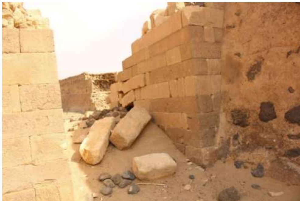
Fig. 27: Al-Mabna dam (Al-Jaufainah) after the lower stones of its drainage channel had been removed (M. al-Ḥajj, 2021).
