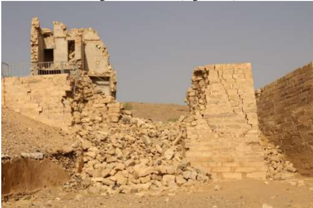
Fig. 24: the upper part of the northern sluice of Ancient Mārib dam after being exposed to shelling (M. al-Ḥajj, 2021).
