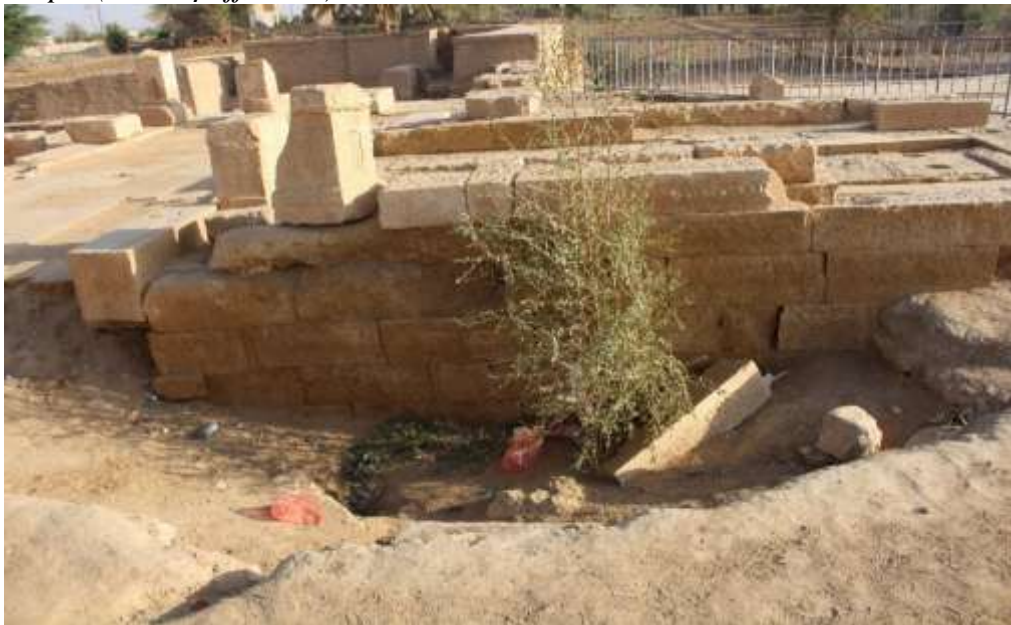
Fig. 22: collapse of the ground of platform in Bar'ān temple, which is located behind the platform of the six columns, and its collecting of rain waters, which may lead to loose of the temple's walls and the platform of the columns in the future (M. al-Hajj, 2021).
